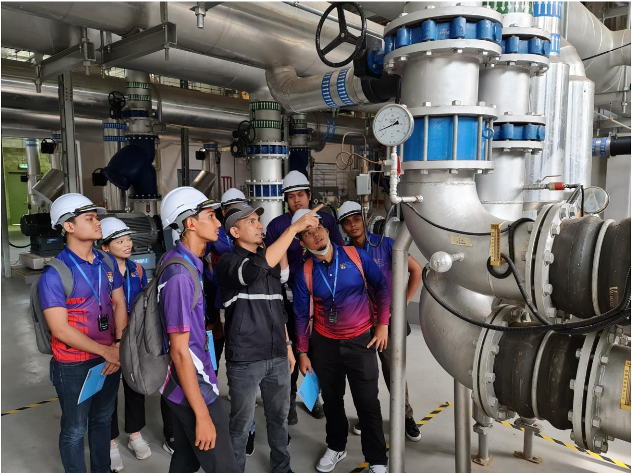
Photo – Dr. Mohd Hafiz Ibrahim, General Manager of Megajana Plant (a Member Company of MGA) was explaining about Cooling District System, that supplies thermal cooling energy to connected building within its network via underground Chilled Water (CHW) pipelines to Final Year students from Engineering & Built Environment, University Kebangsaan Malaysia (UKM) during Technical Visit in Cyberjaya.
